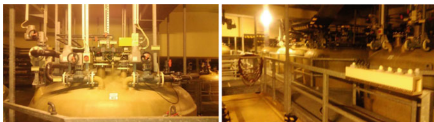
Fig. 2 Reservoir of Decay Tank System (DTS) in Vienna SMZ-Ost Hospital (2 photos, October 2018)
