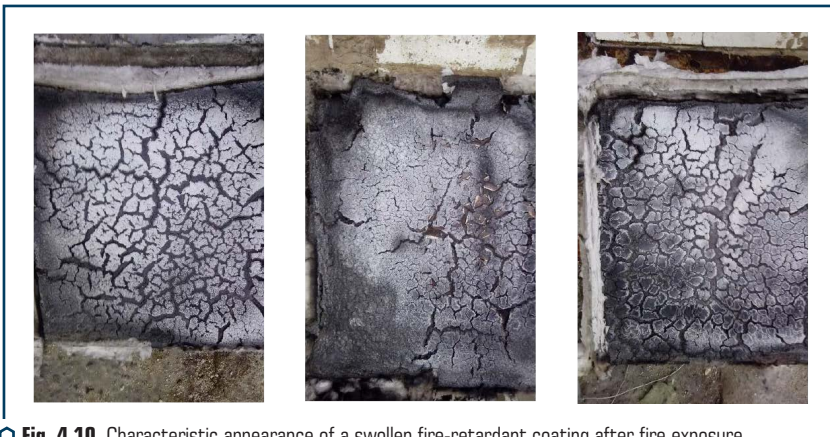
○ Fig. 4.10 Characteristic appearance of a swollen fire-retardant coating after fire exposure
