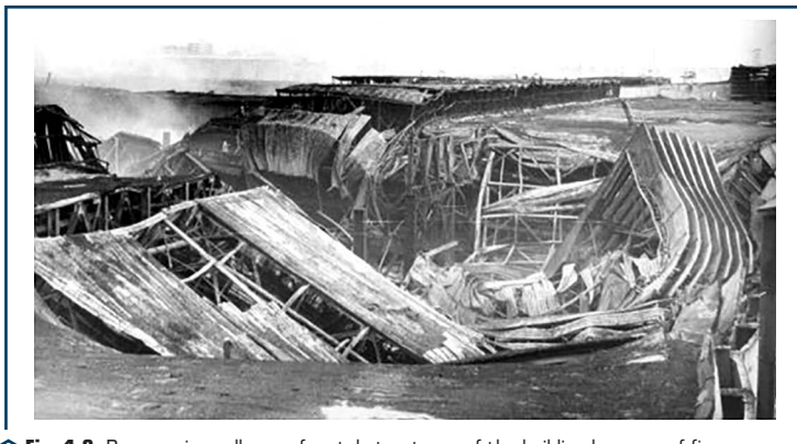
○ Fig. 1.8 Progressive collapse of metal structures of the building because of fire
