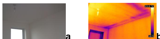
Fig.4. The identification of missing insulation around the MVHR duct: a - the intake duct for the MVHR unit is located above ceiling level in the corner of the room; b - reduced surface temperatures at ceiling level indicate that the duct is not properly insulated
