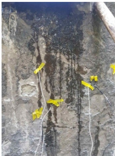
Fig. 5. Small fragment of reinforced concrete wall after the test
