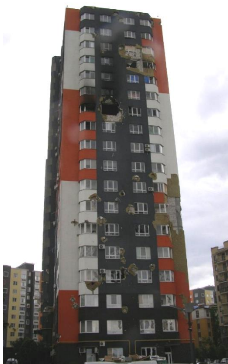
Fig. 1. Facade of the building that has undergone partial damage.
