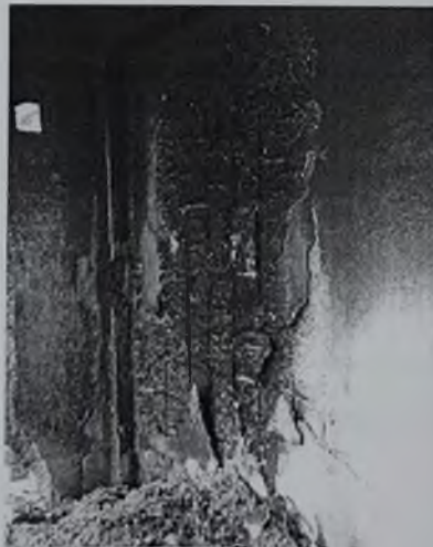
Fig. 2. Nature of structural damage
