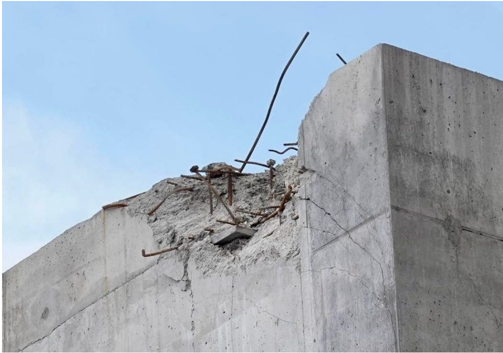
consequences of a combat drone impact on the protective structure
