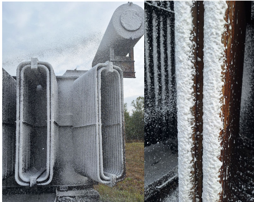
Fig. 3. Appearance of the foam generated from the sodium polyacrylate-based FEA applied to a vertical surface.
