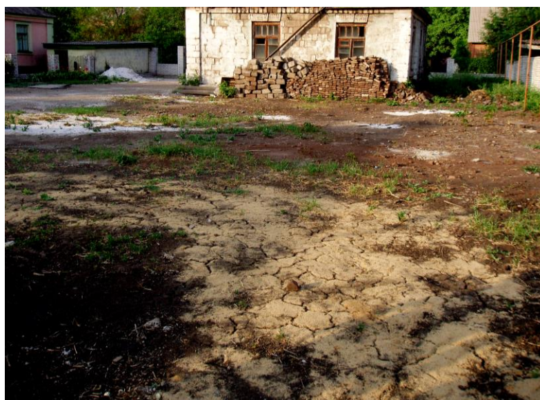
Fig. 1 – General view of area of inspection of the ground foundation, with by the clearly expressed superficial cracks
